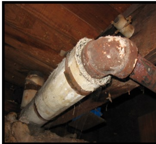
Asbestos Pipe Insulation
