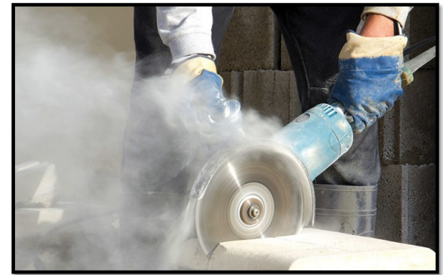
Saw Cutting Concrete Creates Silica Hazard
